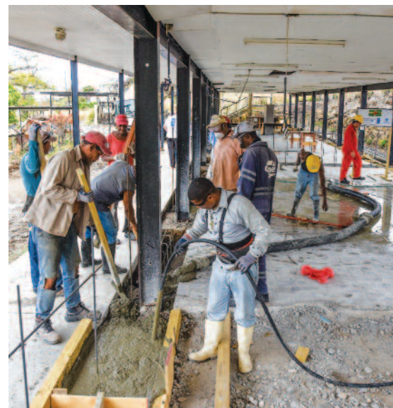
Workers utilizing a concrete pump to pour the concrete foundation for the Salisbury Educational Facility in Dominica
