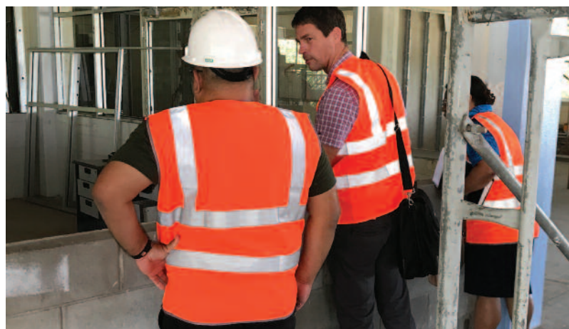
Construction of the Centre for Excellence in Information Technology in the University of Papua New Guinea
