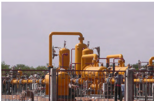
Gas regulator station
