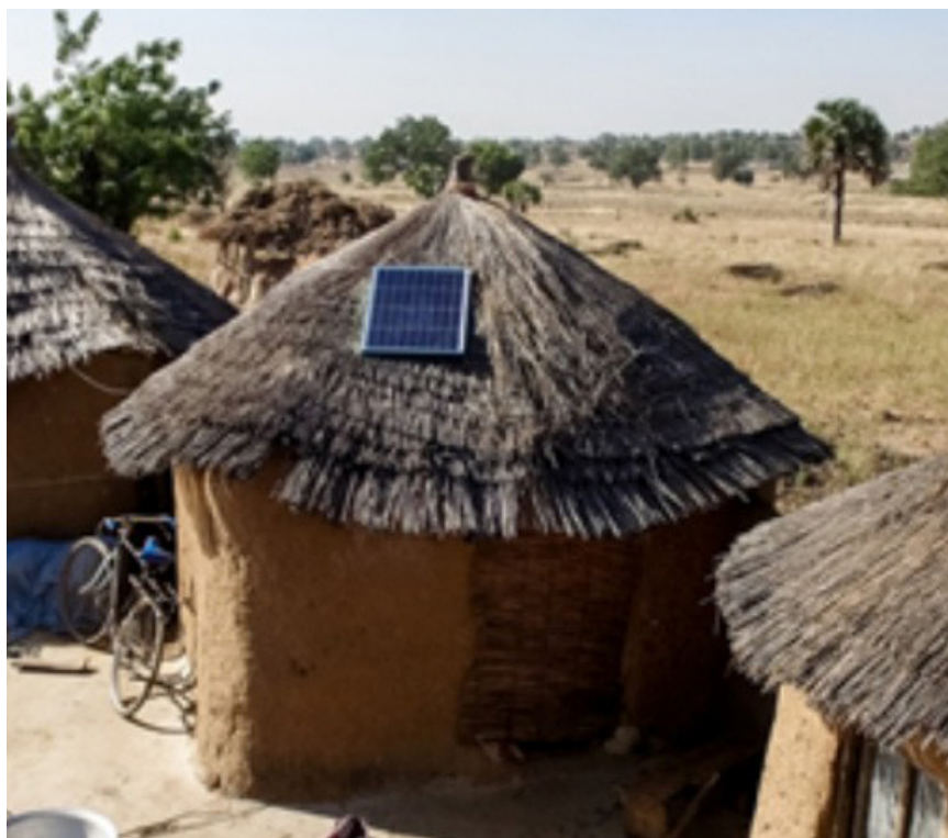
Solar panel on thatch
