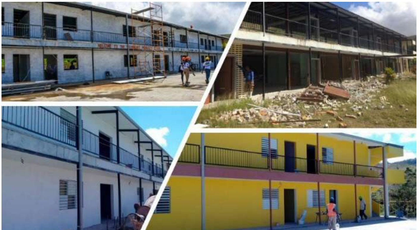
Salisbury Education Facility before and after the hurricane
