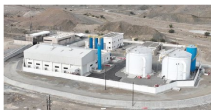
Pumping Stations on the pipeline route
