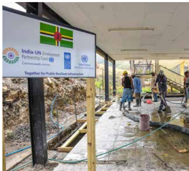
DAMAGE AND RECONSTRUCTION AT SALISBURY SCHOOL COMPLEX
