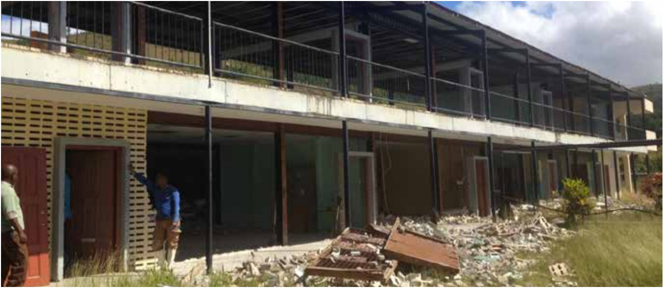
DAMAGE AND RECONSTRUCTION AT SALISBURY SCHOOL COMPLEX
