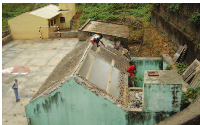
Dilapidated health-care centre before refurbishment
