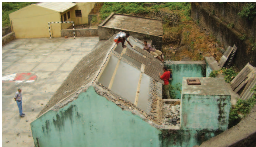
Dilapidated health-care centre before refurbishment
