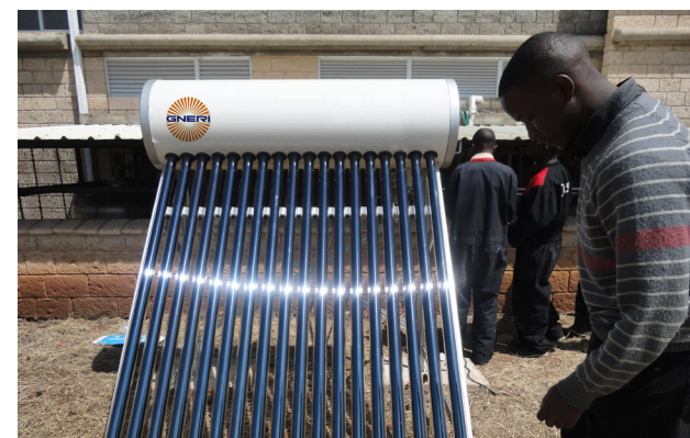
Left: Solar product donation ceremony by GNERI/UNIDO-ISEC in Thika, Kenya; Right: Solar water heater demonstrated in Kenya
